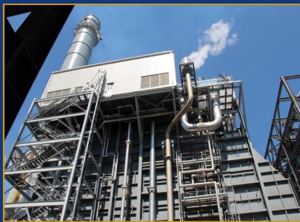
Duke Energy's gas-powered plant, Masontown, Pennsylvania.
