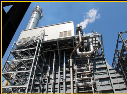
Duke Energy's gas-powered plant, Masontown, Pennsylvania.
