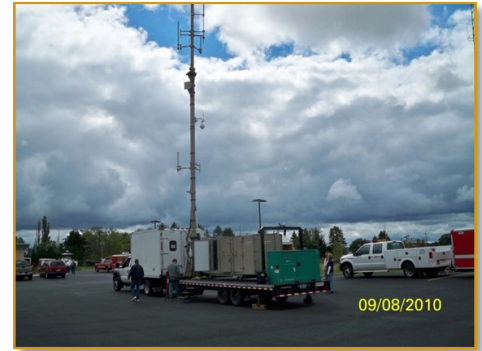
Cell on Wheels ensuring reliable emergency communications.
