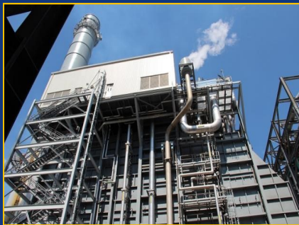
Duke Energy's gas-powered plant, Masontown, Pennsylvania.
