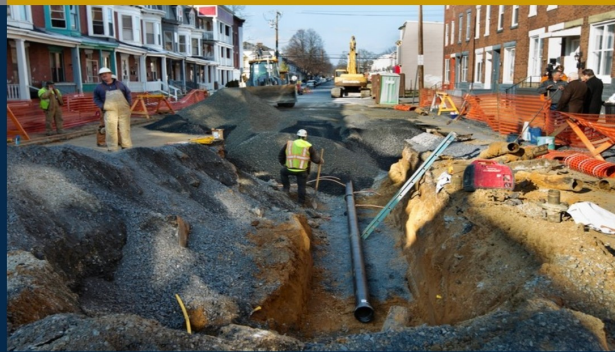
Harrisburg City: 1st sink hole mitigation project using FEMA, Pre-Disaster Mitigation Grant funds in the nation
